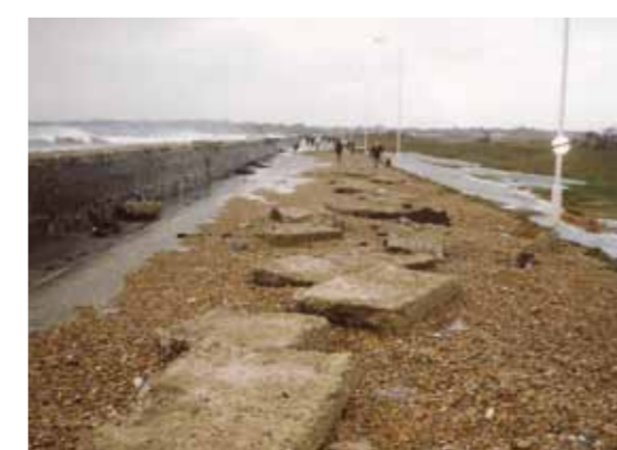
Damaged sea wall after a storm on Preston Beach Road, Weymouth.
